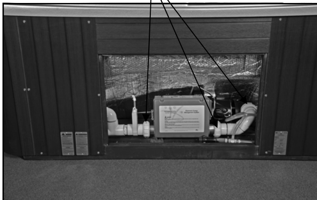
...THROUGH THE PUMP UNION
